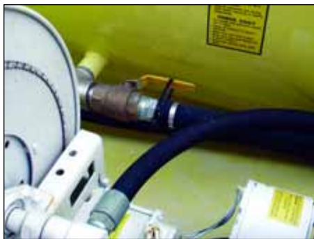
Safety valves are typically located at the outlet of each tank, and in front of each hose reel. Zip-ties used to hold the valve in the open position can be slid back and the valve closed should the need arise.
